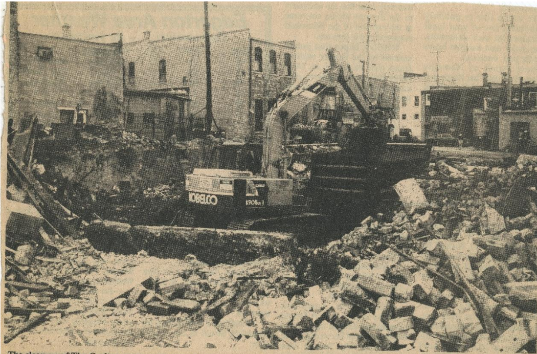
The clean-up of The Carlton continued last week. Currently the site is clear and the hole has been filled in. The investigation into the fire continues. The official cause is still undecided. Investigators are awaiting the outcome of lab tests that are being done on the evidence gathered at the scene.
