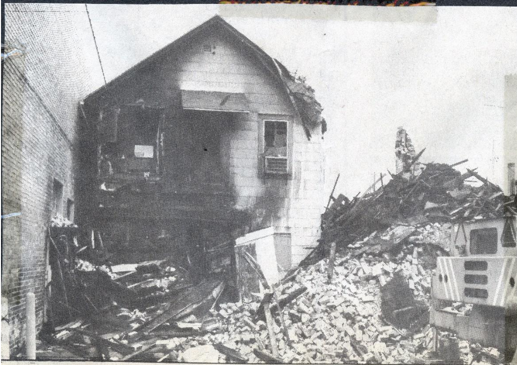
The rear of the building which housed Mildred's Antiques was destroyed by the fire.
