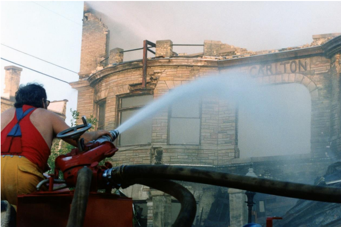
Carlton Hotel Fire – September 9, 1991:
